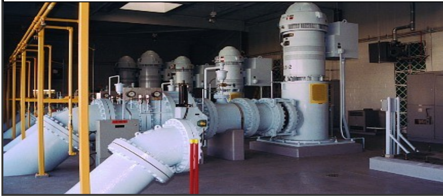
Water Pumping Station
